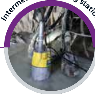
Water Recovery / Intake
