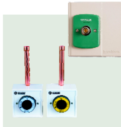
Gas outlets: plug in for any gas
