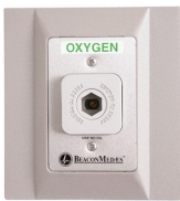
Medical gas outlets
