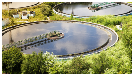
Waste Water Treatment
